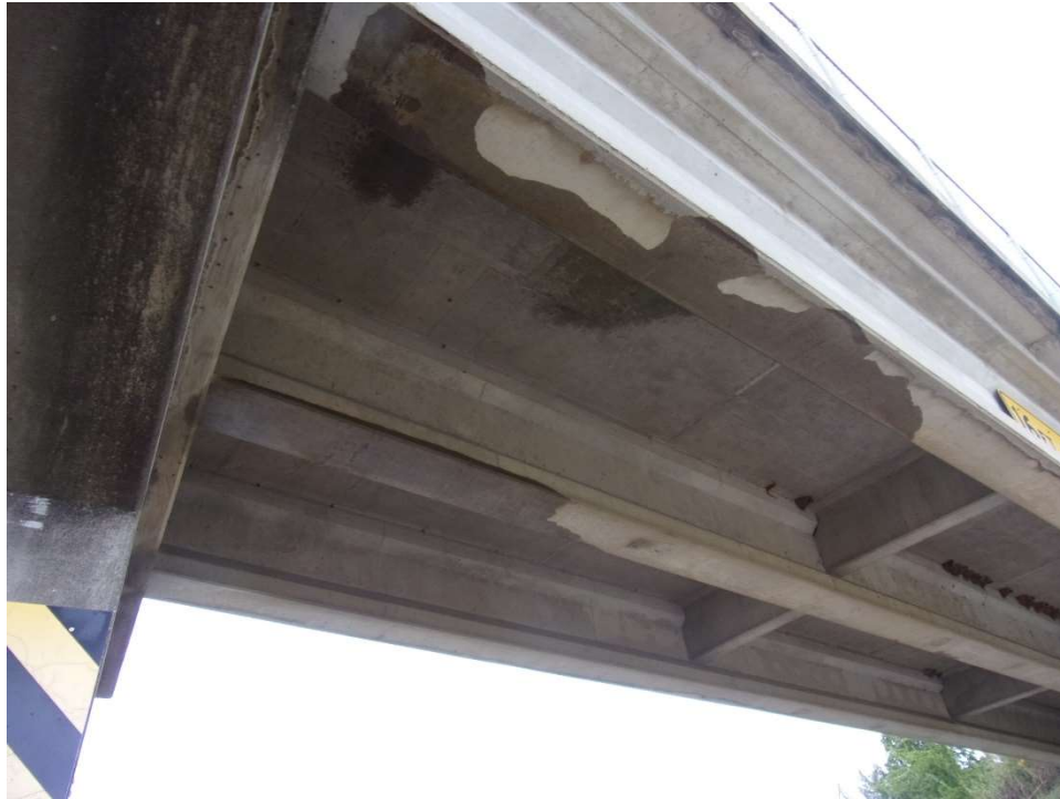
Photo 8: Diesel Fuel on Beams
