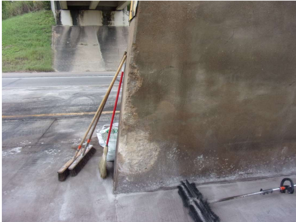
Photo 3: Spalled Concrete on North Side of Pier
