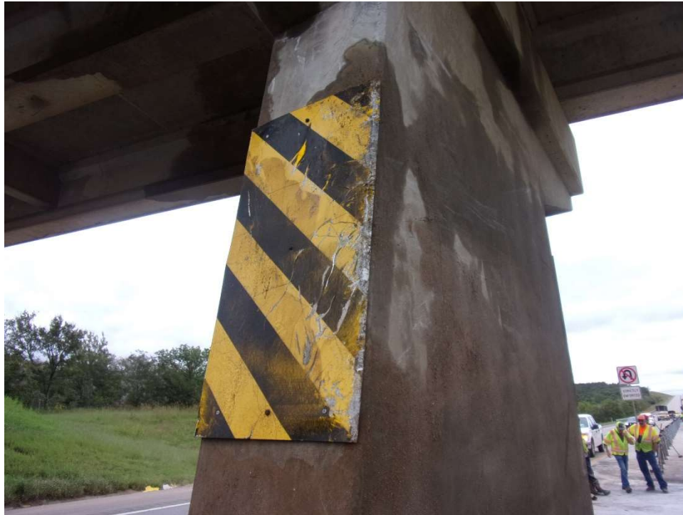
Photo 6: Damaged X-3 Marker
